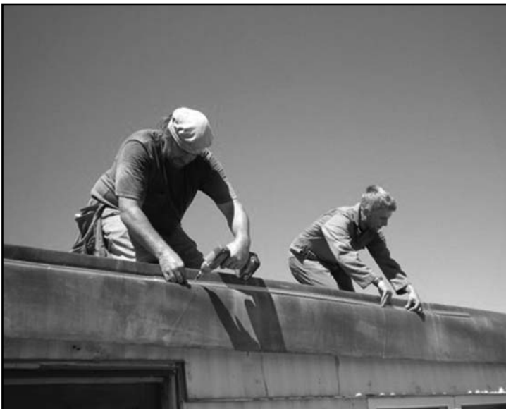
Scott Hessel, CSC Weatherization Crew Leader, and a weatherization student apply a roof to a mobile home.
