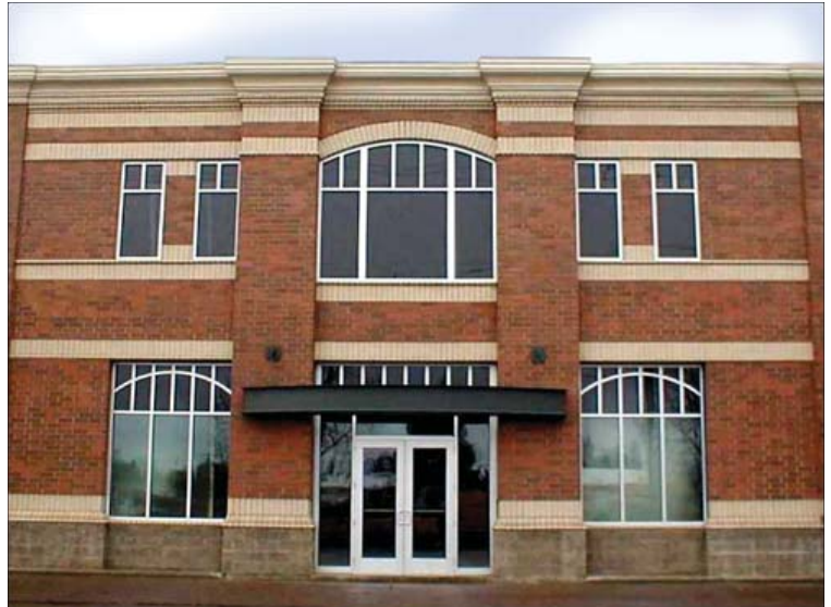
The restored facade of Woodburn's Association Hall, funded, in part, by the Small Community Incentive Fund.
